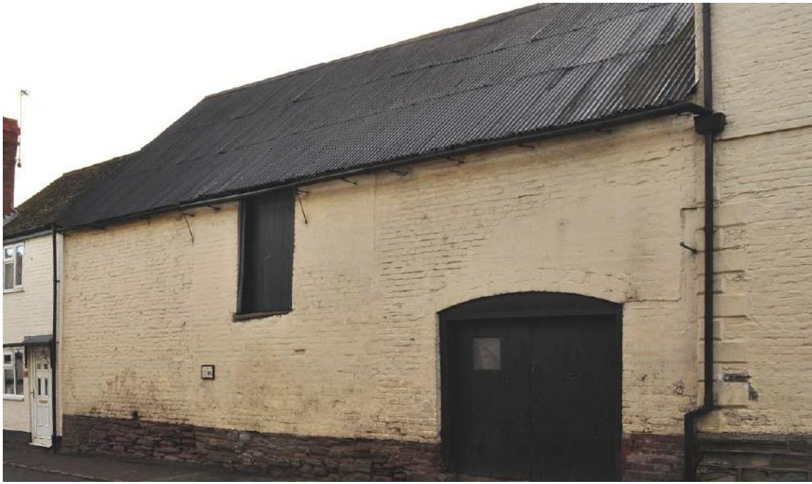
Figure 4: Subject barn prior to conversion showing an absence of openings to the roof slope
